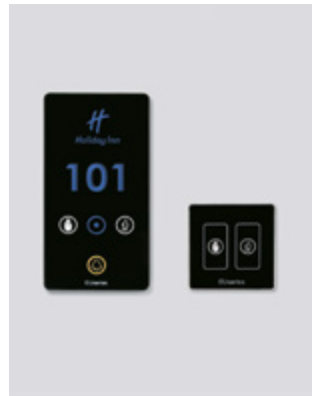
Occupied room (indicator panel & in-room panel)
